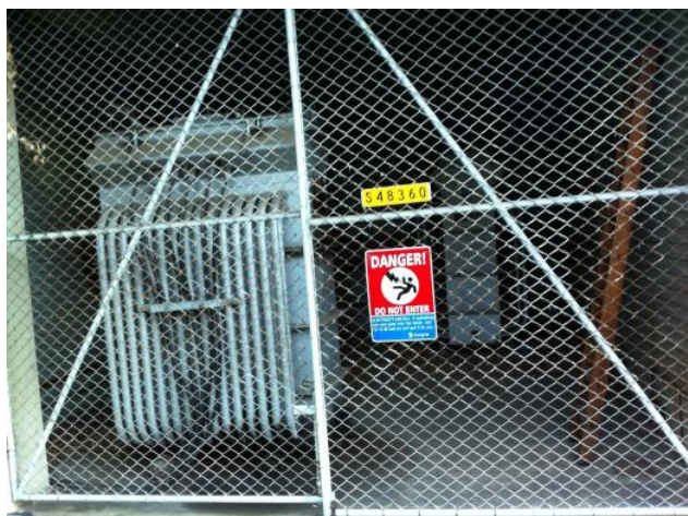
Photo 5.9.2 – View of the Transformer room and the staining of floor at the bottom
