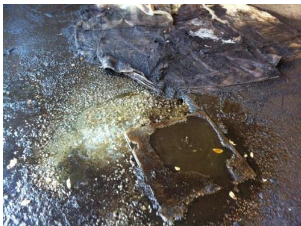
Photo 5.3.7 – Staining of concrete floor and the hole in the concrete in the grout area
