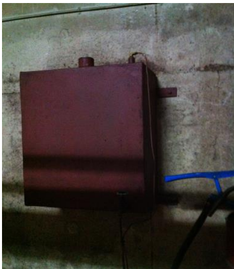
Photo 5.5.3 – 80L diesel AST in the northern pump room
