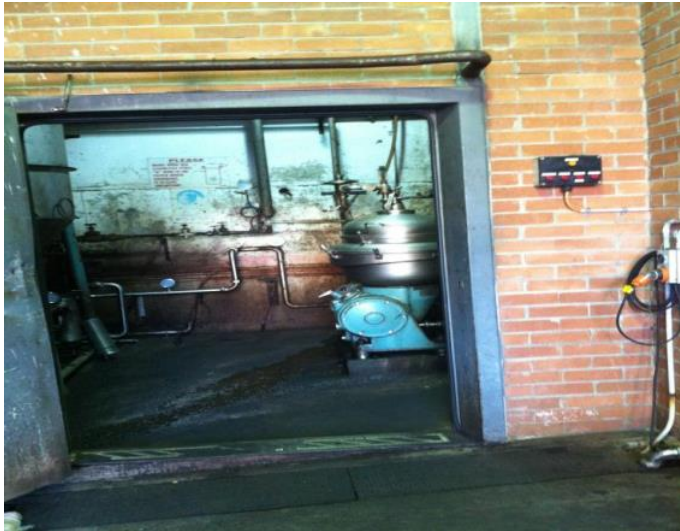
Photo 5.3.8 – Oil-water separator room
