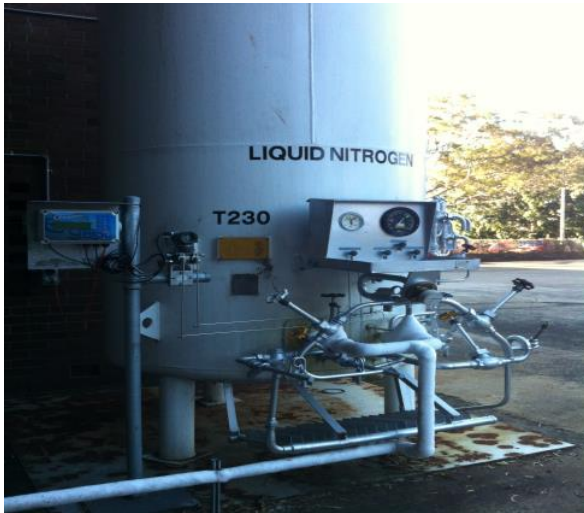
Photo 5.5.1 – Liquid nitrogen AST
