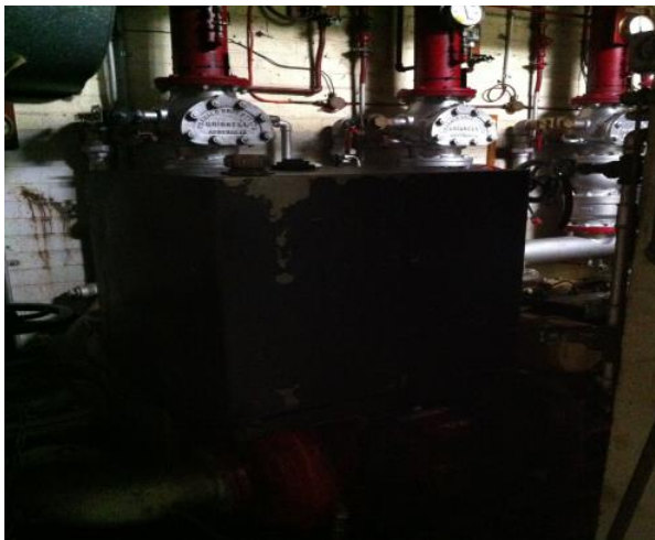
Photo 5.5.2 – 80L diesel AST in the southern pump room
